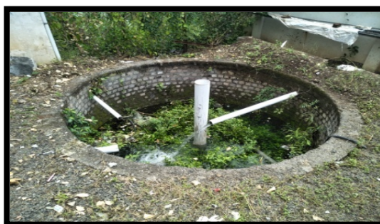
Fig.7.3 Water Recharge Tank
